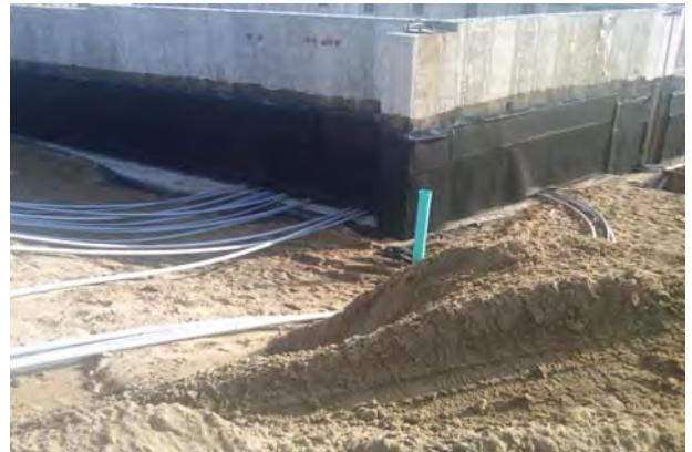
Electrical conduits in basement area
